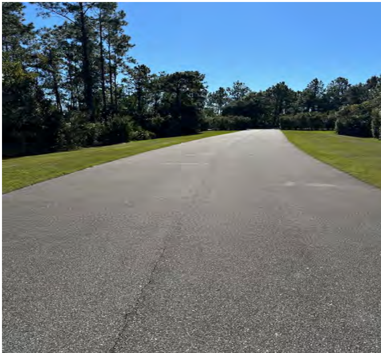
View from middle of road at midway point looking from Glorieta Drive to Vale Drive
